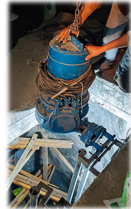
Marina Project Pumps
